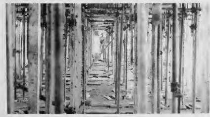
A maze of pipes used to support a poured concrete roof forms a confusing jungle as an addition to the colony high school is erected. Three hundreds of supports will be removed when the reinforced concrete slabs hardens. In the meantime, it's an intricate jeh for the concrete workers of the Masons and Insulators.
